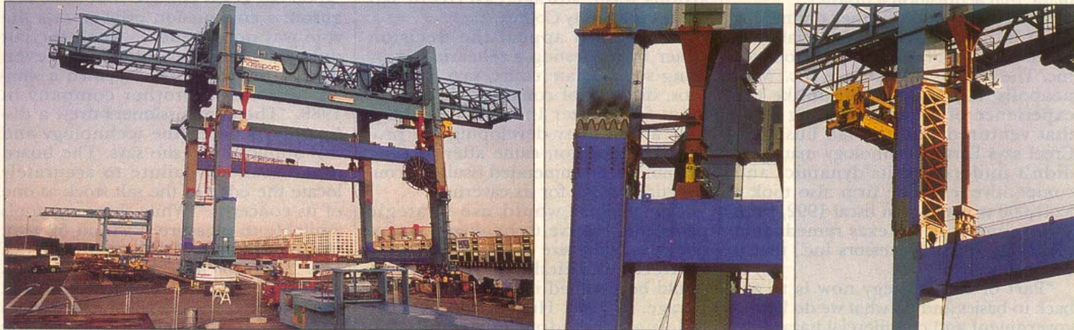
New portal beams, painted blue, were installed, and jacks were based on them (center photo). Holes in telescoping sleeves welded to crane legs above the cut enabled it to be temporarily bolted to leg if crane was needed. Temporary cross bracing, installed as jacking proceeded, was replaced with plates.
